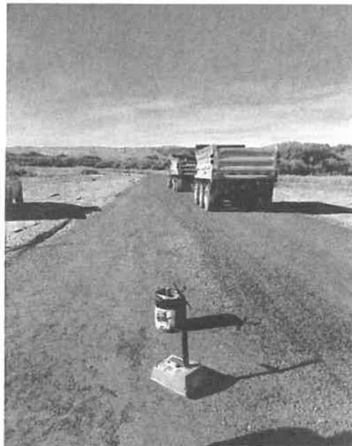
Performing Density testing of Base Course Subgrade on Dapple Gray Way Rd. (Ref. Test #1 above)
