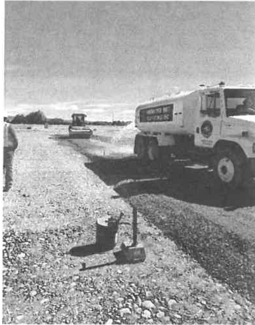
Compaction applied via Drum Roller near Dapple Gray Way and Roan Rd. Southern Intersection.
